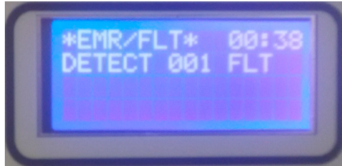
Figure 25) Typical FAULT state screen.
